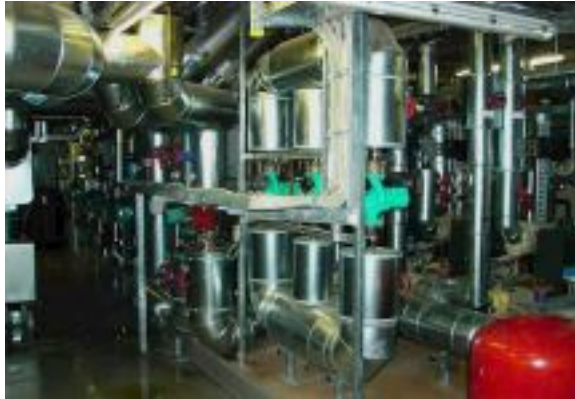
Cooling plant, Medical Institute Düsseldorf, Germany View image
