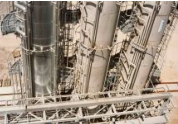
Refinery MIRO GmbH, Karlsruhe, Germany View image
