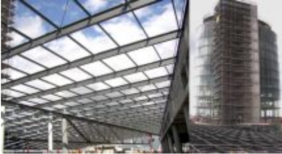
DaimlerChrysler AG, New Branch Munich, Delivery and assembly of completely welded construction View image
